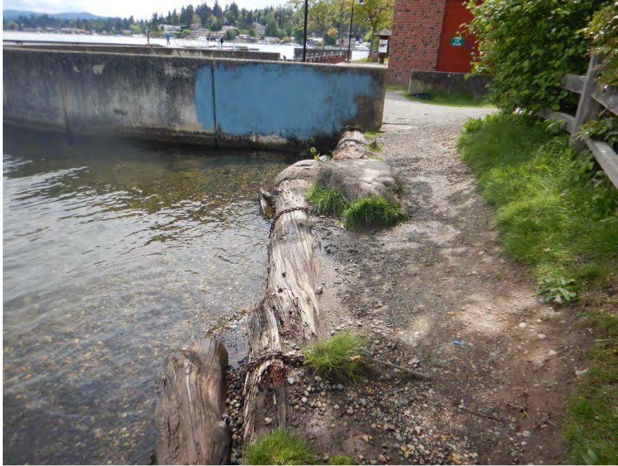
Photograph 9. Looking south from north beach toward existing bulkhead and Boiler Building (May 2022).
